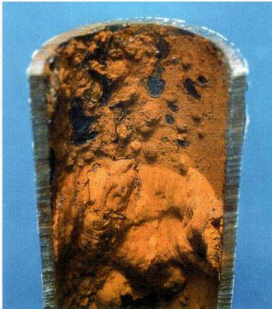
Galvanized pipe heavily corroded.
