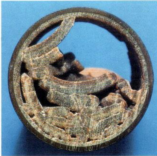
Copper pipe with scale plug.
