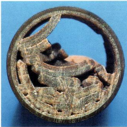
Copper pipe with scale plug.
