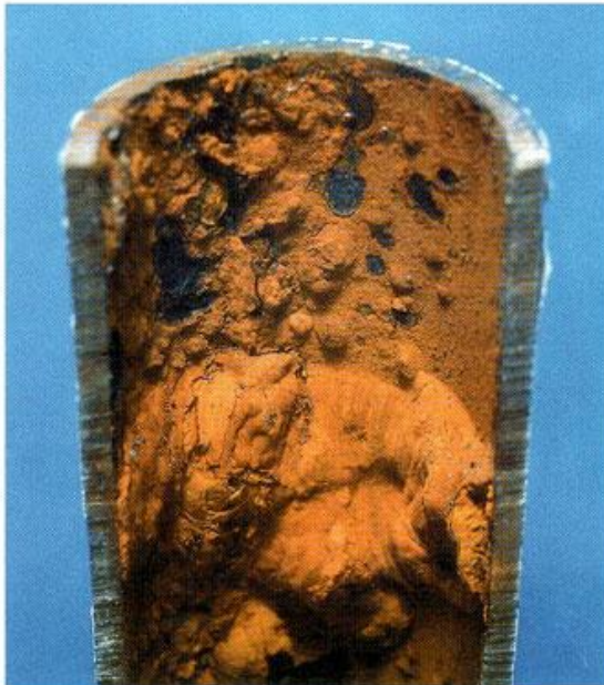
Galvanized pipe heavily corroded.
