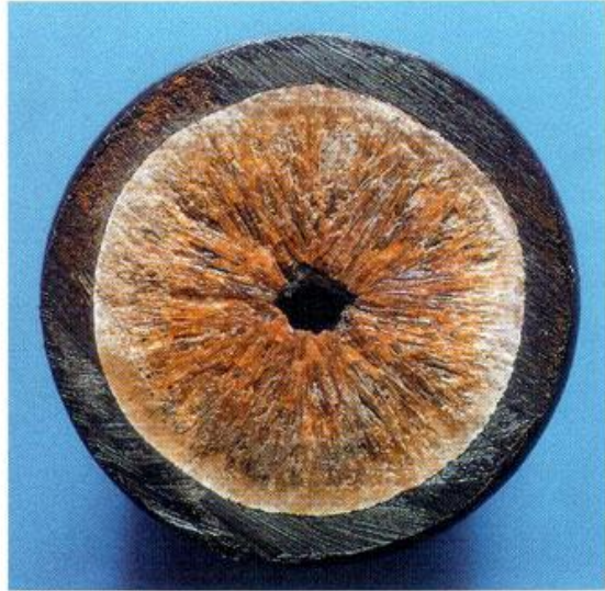
Galvanized pipe heavily scaled.
